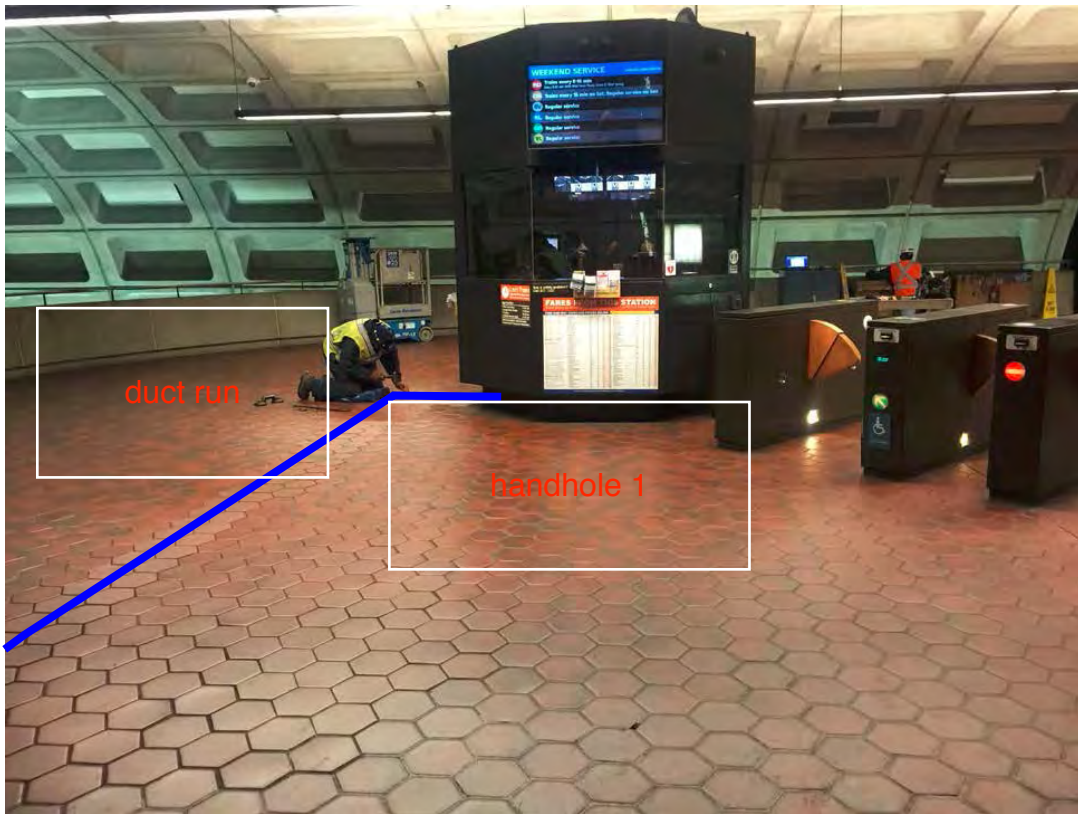
Photo #1 – K03 Virginia Square: Duct run from kiosk to handhole 1
