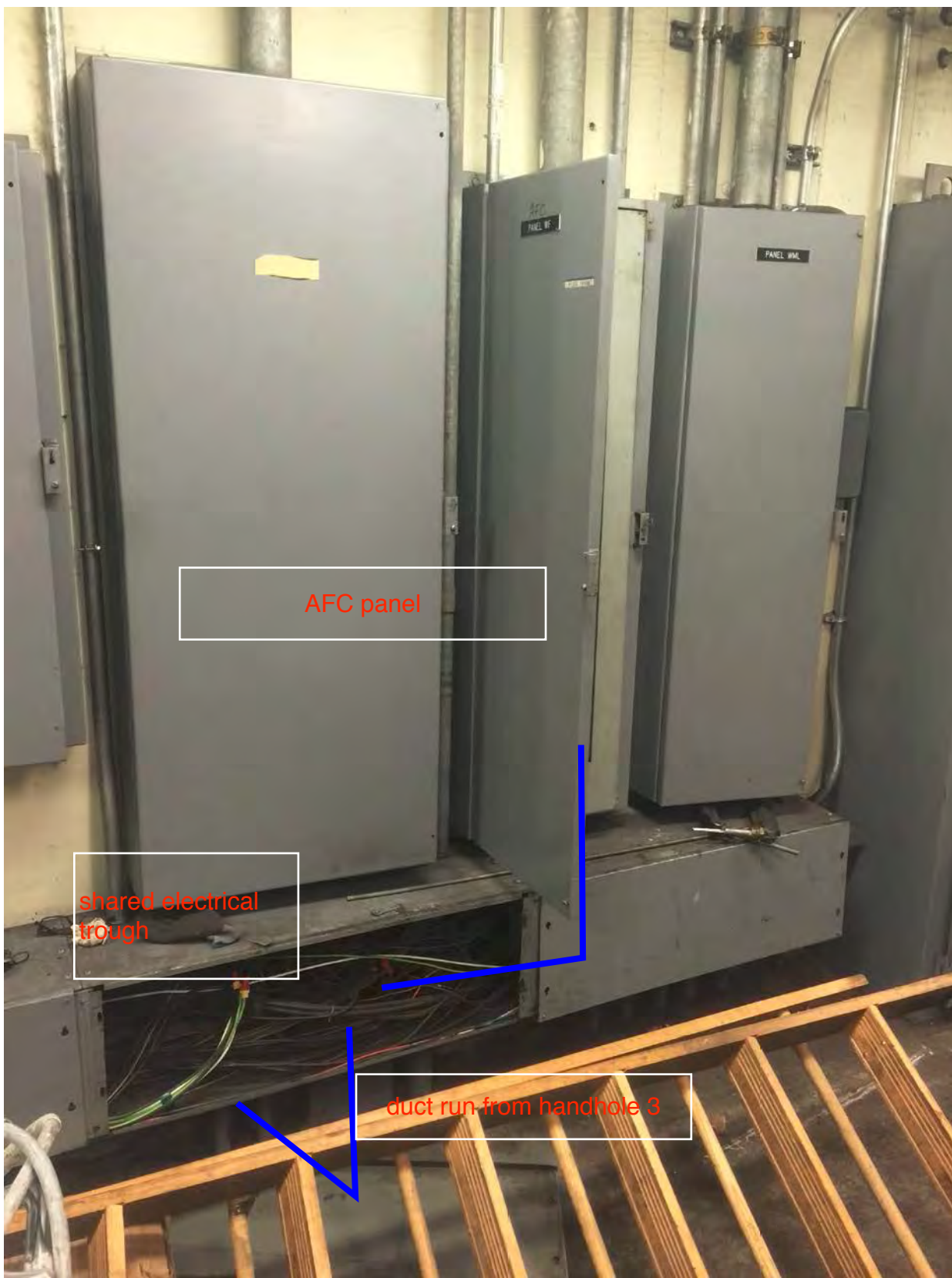
Photo #4 – K03 Virginia Square: Duct into AFC panel from handhole 3
